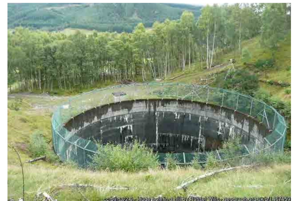
Figure 12 Cluanie Surge Shaft with safety fencing
