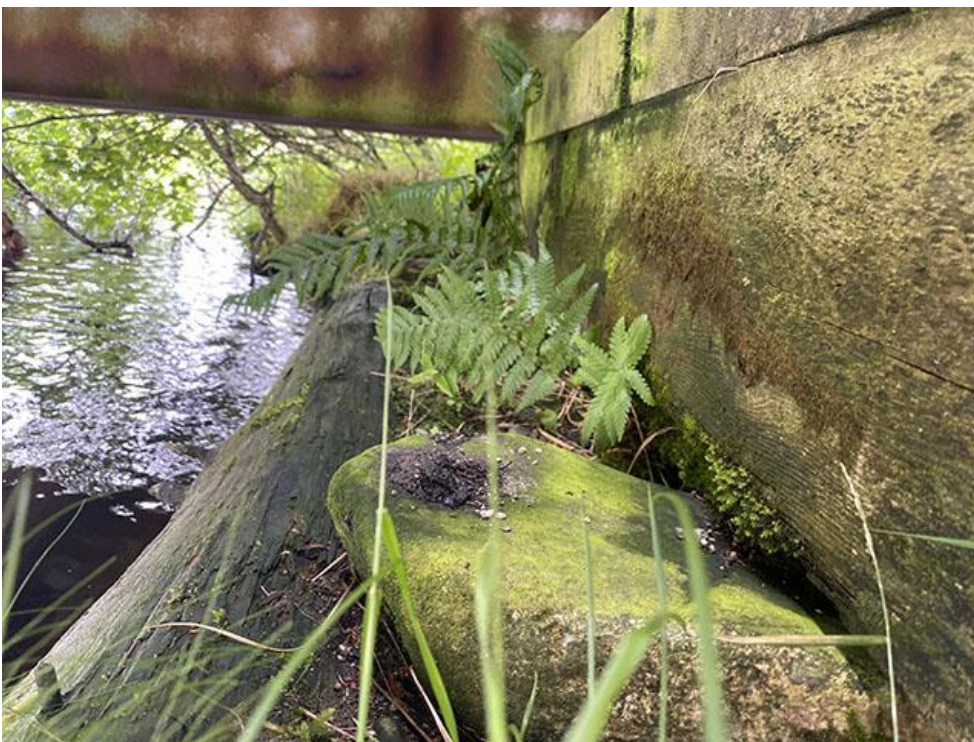
Plate 6: Extensive sprainting beneath both sides of bridge.
